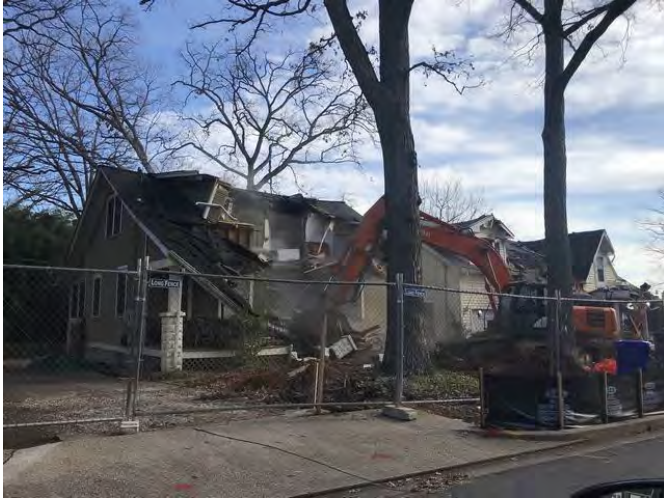
Single-family homes adjacent to the Subject site being demolished to make way for townhome condominiums
