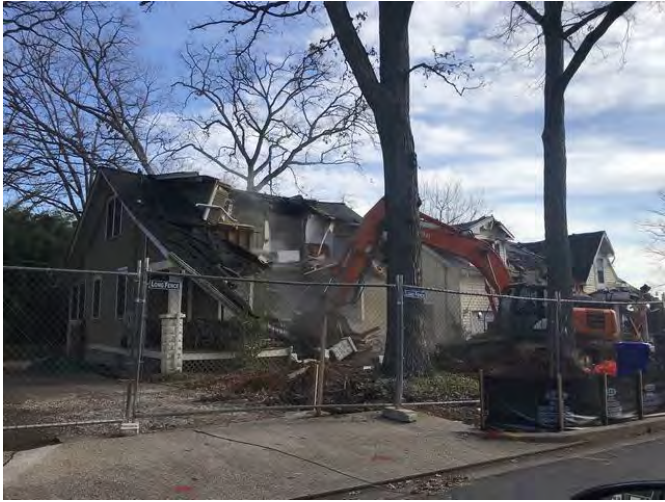
Single-family homes adjacent to the Subject site being demolished to make way for townhome condominiums
