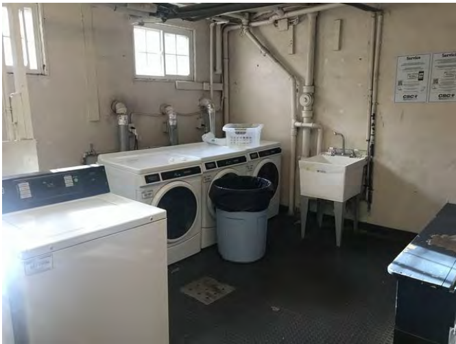
Subject central laundry facility
