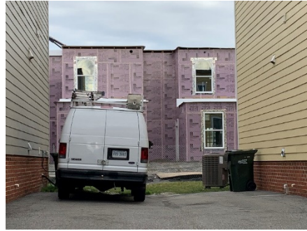
Townhomes at Warwick Place II
