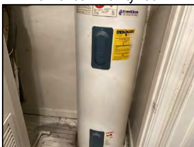
View of typical hot water heater
