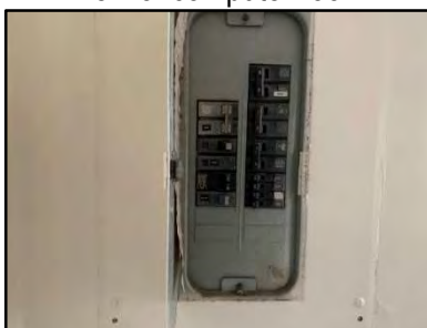
View of typical electric panel in apartment
