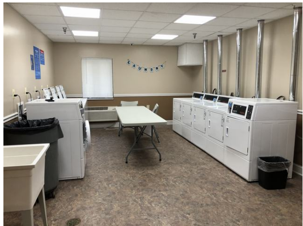
Central laundry facility
