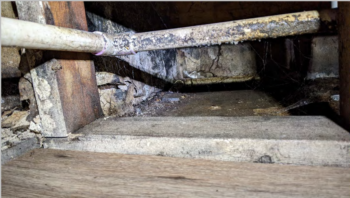
Return Plenums Show Signs of Water Damage and Mold Growth
