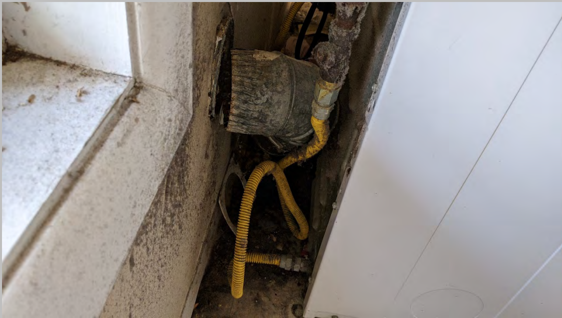
Community Center Dryers are Gas; Also Venting Issues with Connectivity to the Outdoors
