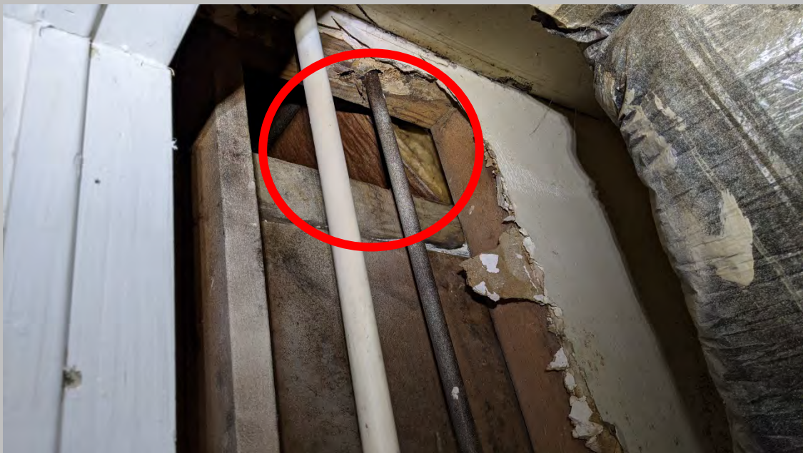
Attics Were Inaccessible Although a Hole in the Drywall Shows an Older R-13 - R-19 Basket Weave Style Insulation (!970's)
