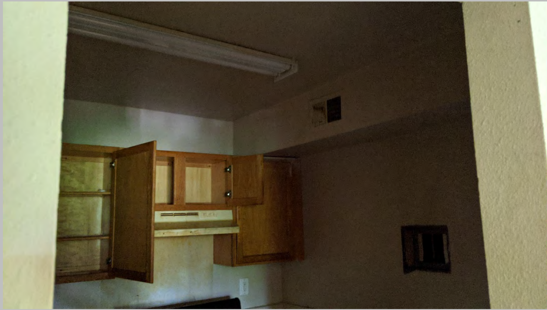
Range Hood Without Direct Outdoor Ventilation
