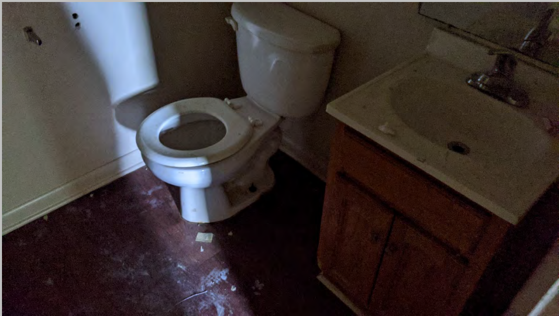
Typical Water Closet and Sink for Dwelling Unit Bathrooms
