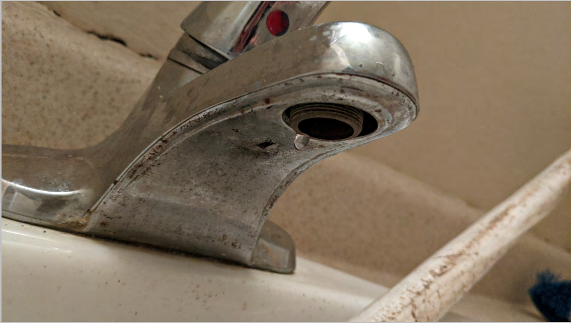
Typical Lavatory (Most Were Missing Aerators)
