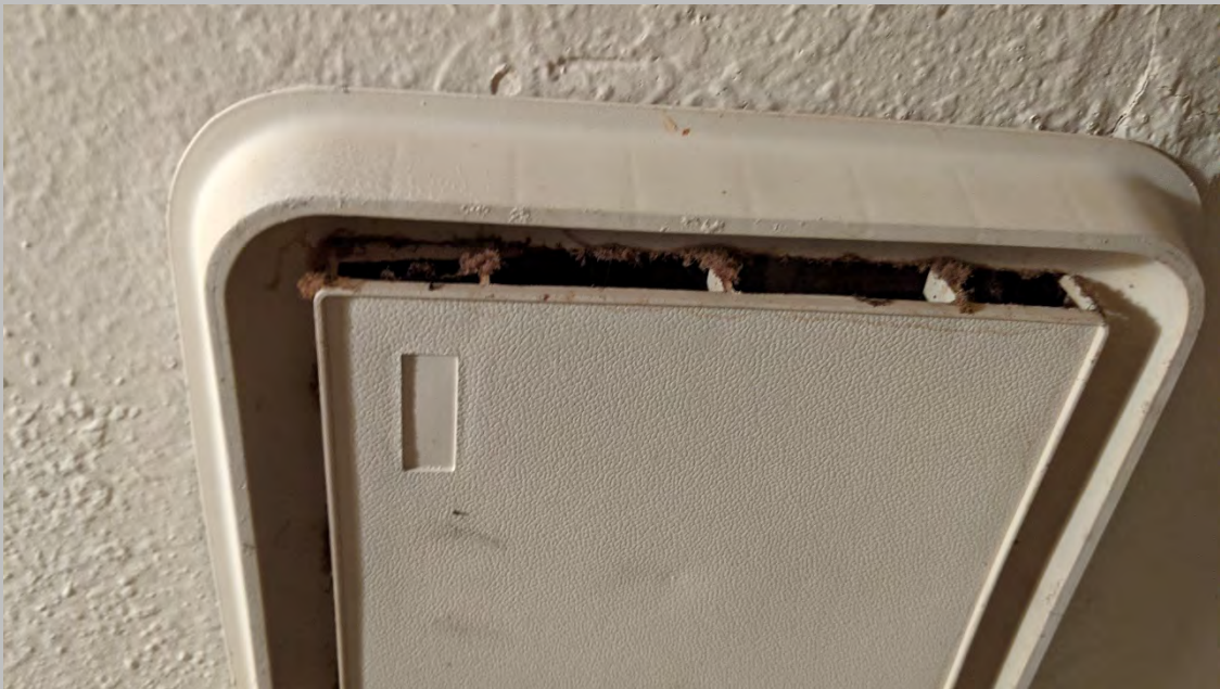
Typical Bathroom Exhaust – Could Not Confirm Direct-to-Outside Venting
