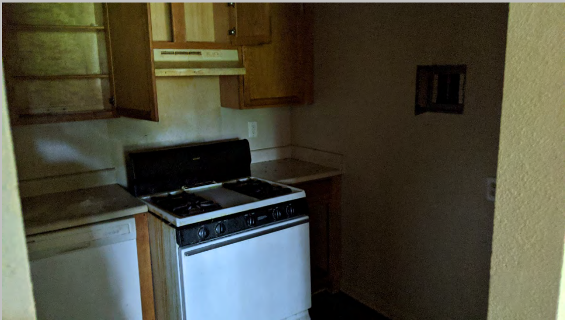
Typical Gas Range at Dwelling Units
