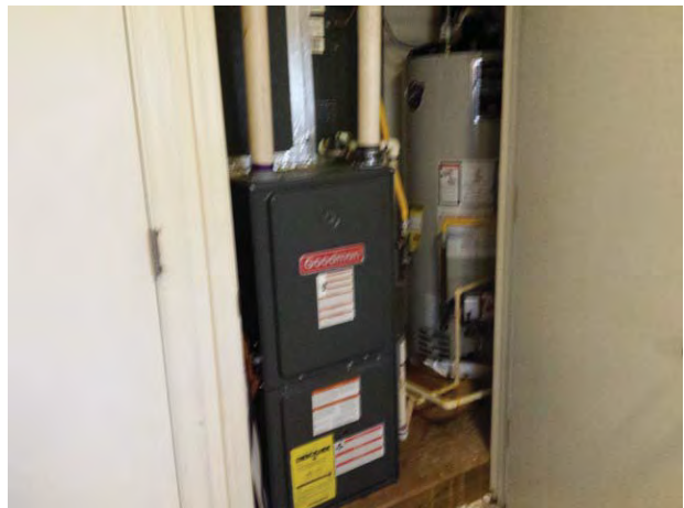
Typical mechanical closet - occupied unit
