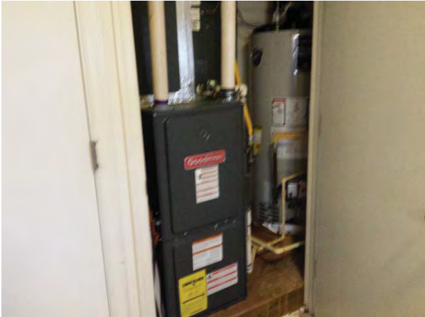
Typical mechanical closet – occupied unit
