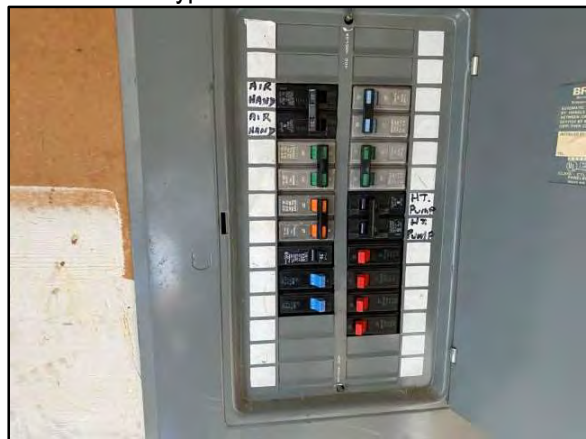
View of typical electric panel in unit
