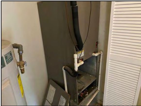
View of typical furnace
