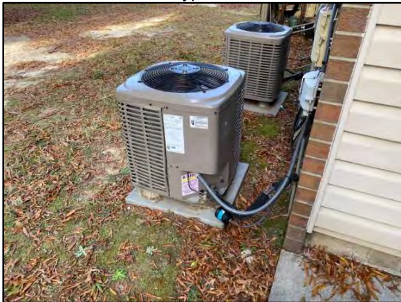
View of typical air conditioner condensers
