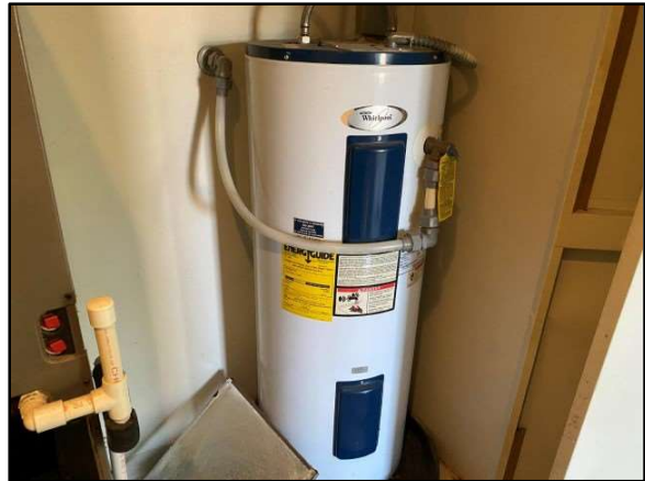
View of typical hot water heater
